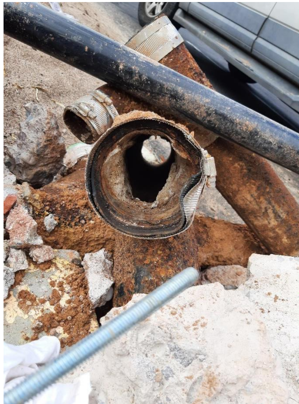
A pipe with significant FOG accumulation
